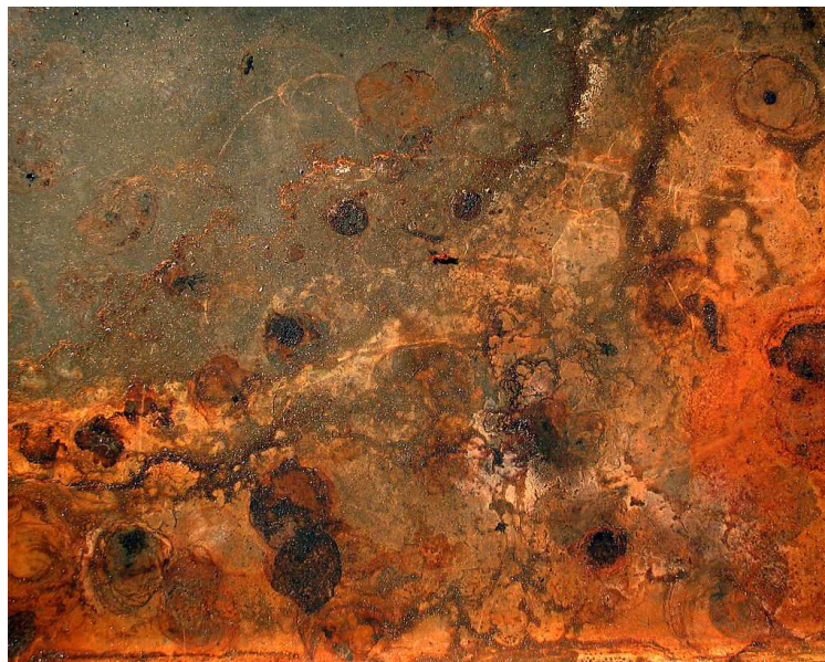
Fig. 15. Rust-The most familiar example of corrosion
